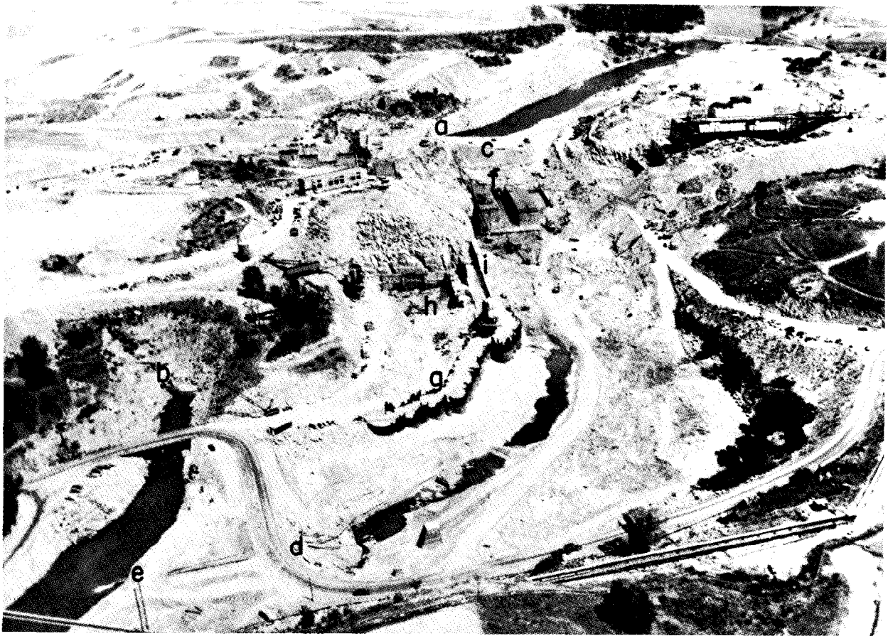
Figure 5-2. Diversion of the river during construction of Folsom Dam and Powerplant in California.-AR-16270.
