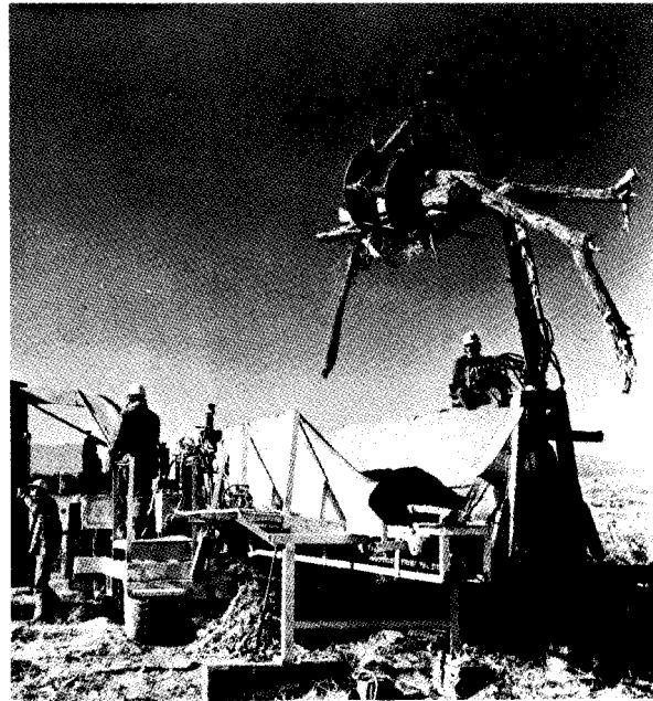
Figure 15-9. Chipping operations at Pueblo Dam in Colorado. All brush and timber smaller than 7 inches in diameter are chipped and stored for use as a mulch on reseeded areas.—P382-700-790 NA
