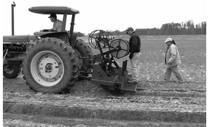
Figure 3. Custom-made dripline installation tool is shown in the top diagram (courtesy of F.R. Lamm, Kansas State University); installing dripline with commercial installation tool is shown in lower photograph.
