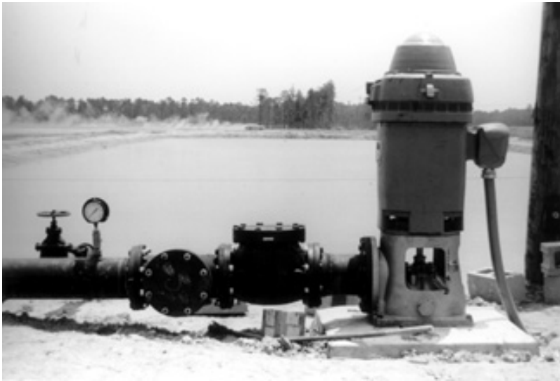
Figure 14. Large agricultural well with electric motor
