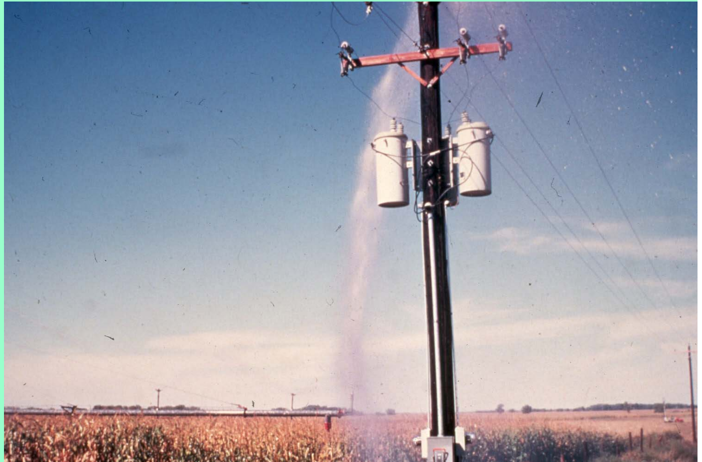
End gun spraying power lines & transformers
