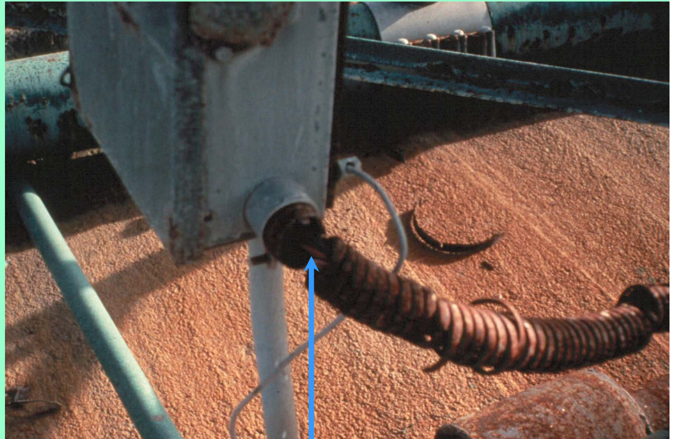
Old Corroded & Broken Conduit
