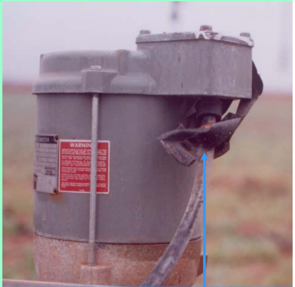
Cord Damage With Tape Coming Off
