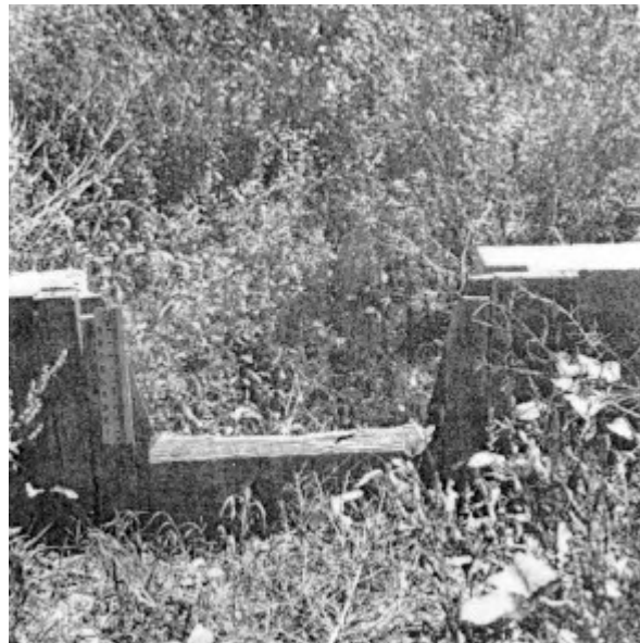
Figure 5-8 -- Poorly maintained weir edge.
