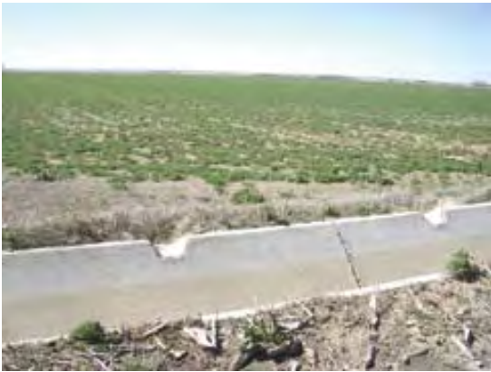
Border/basin check outlet
