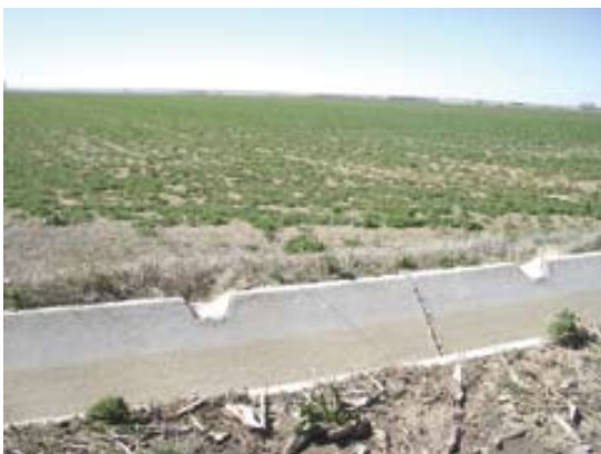
Border/basin check outlet
