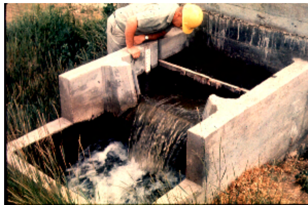
Figure 7-11 -- Weir box turnout with Cipolletti weir.
