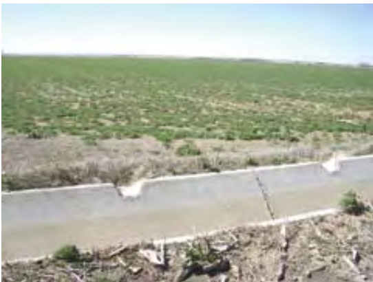
Border/basin check outlet
