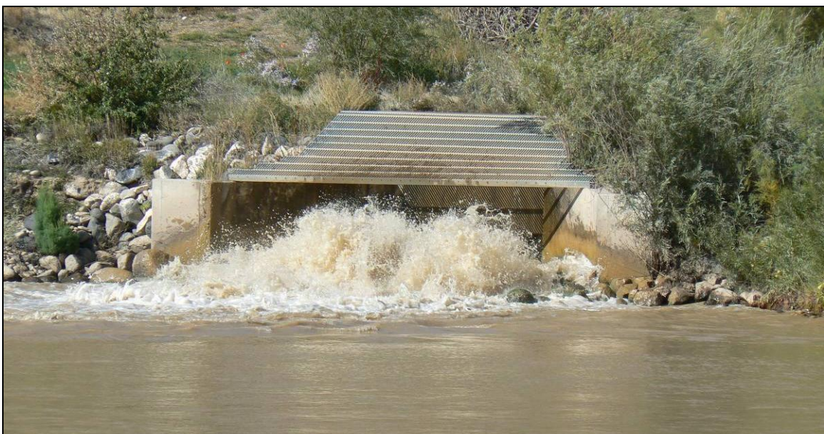
Figure 3: Pipeline Spill Returning 75 cfs to the Colorado River
