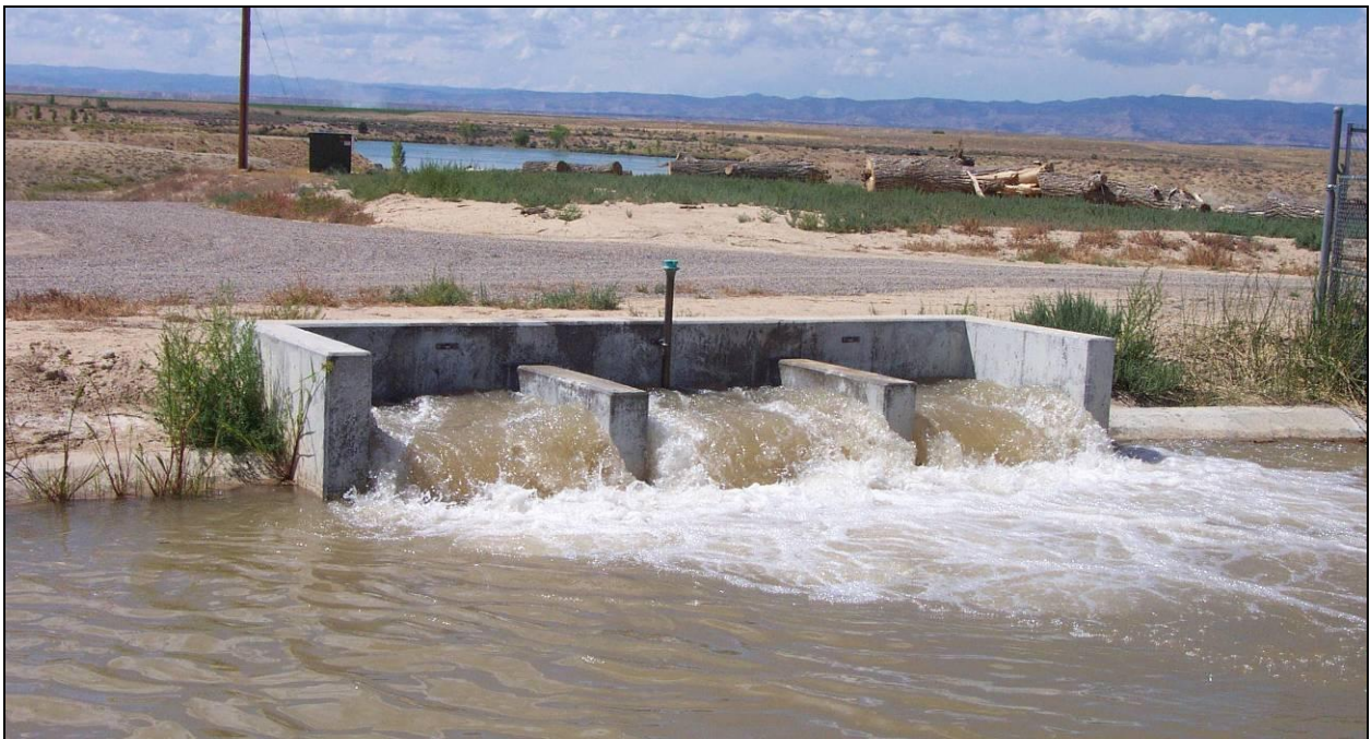
Figure 6: The Pump Station Delivering 70 CFS into the Highline Canal
