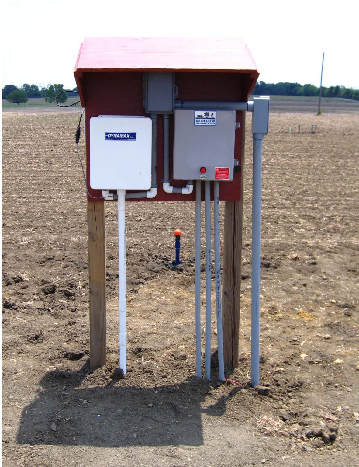
Figure 7. Finished field experimental system (Datalogger and Control box) at Black Belt Research and Extension Station, Marion Junction, Dallas County, Alabama.
