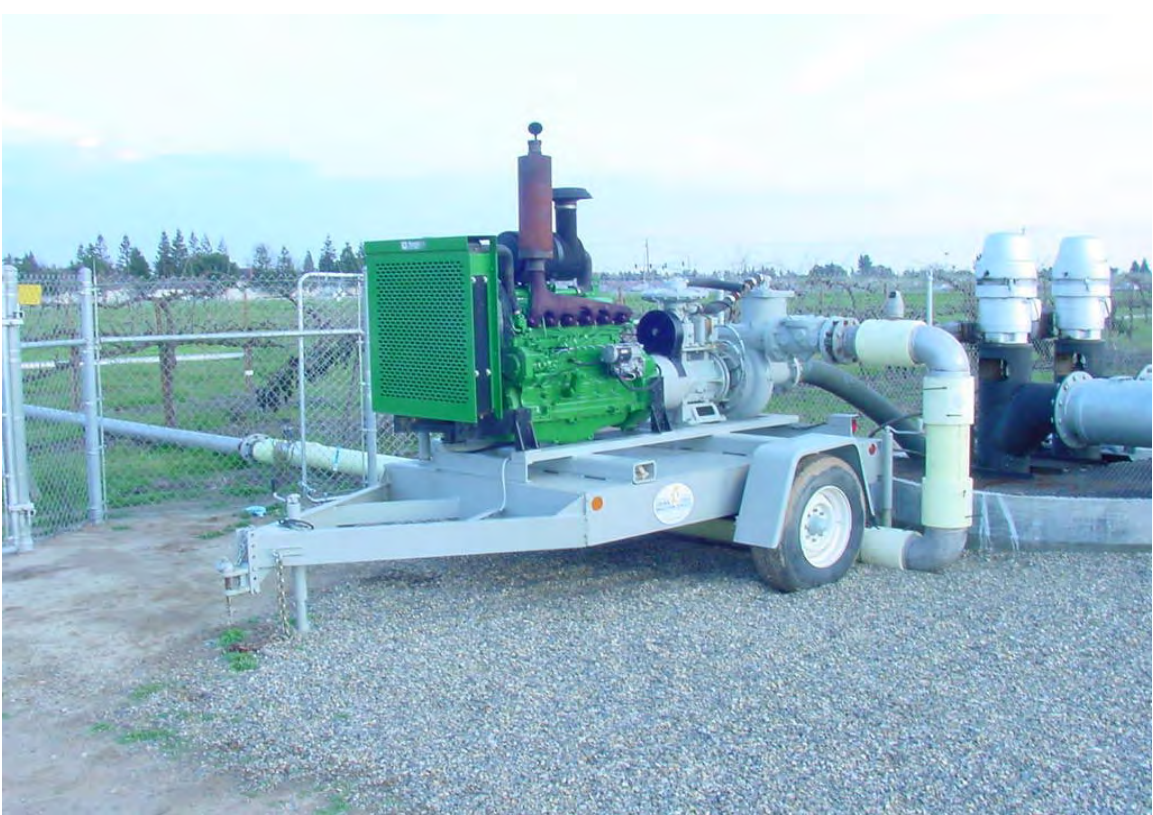
Figure 3 Portable pumping plant. Note the water meter is visible in the 8 inch mainline just outside of the security fence.
