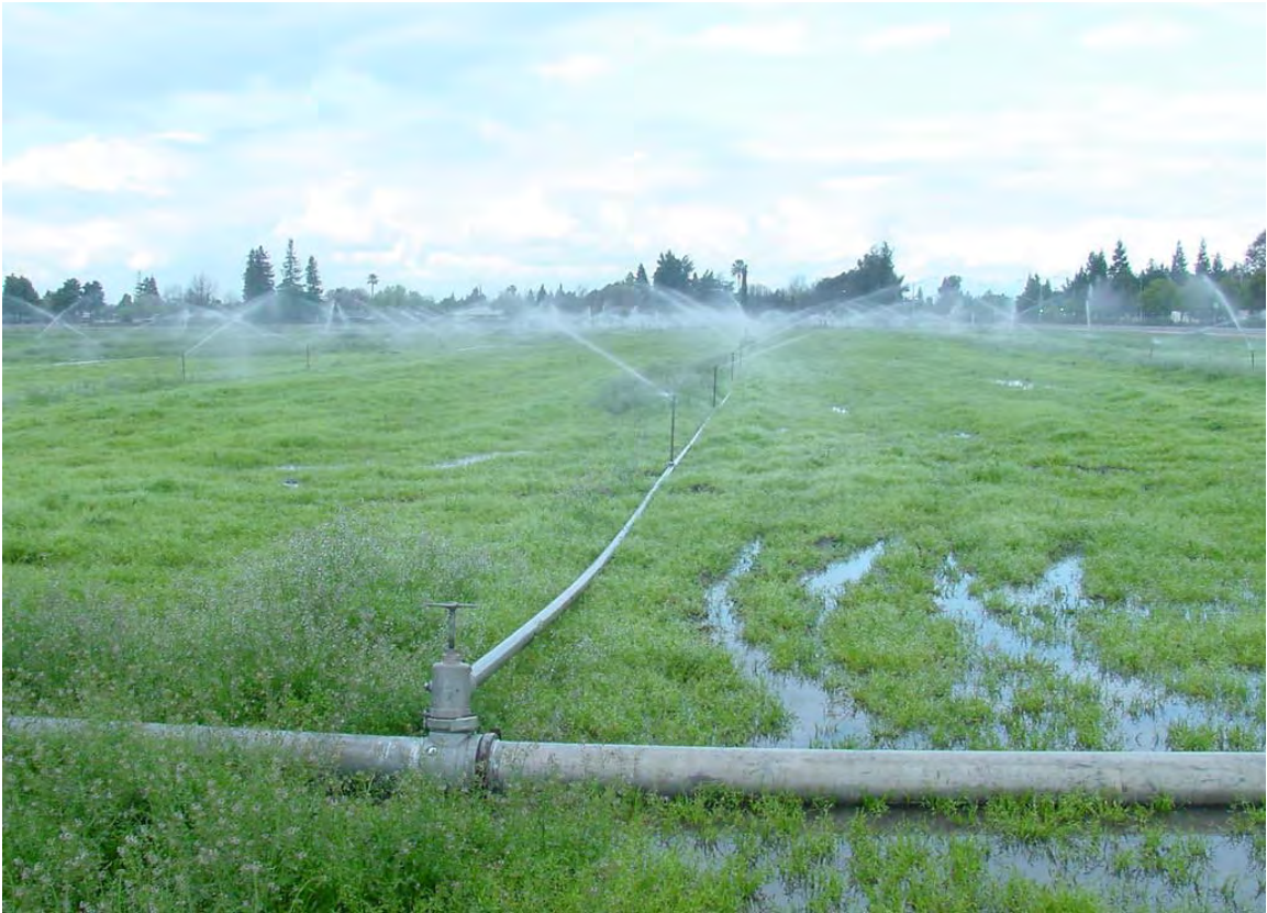
Figure 1 Portable aluminum pipe solid set system in operation.
