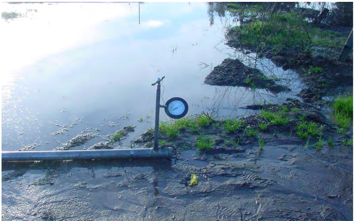
Figure 4 Pressure gauge mounted on a riser at the end of the lateral.
