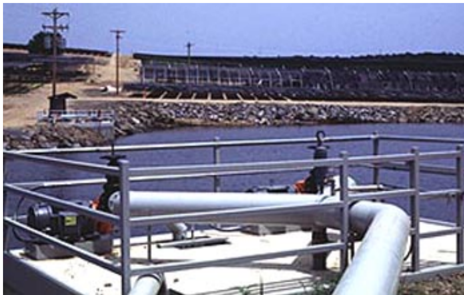
Shown here is a retention basin for capturing irrigation runoff and equipment for pumping captured water to a storage pond at a higher point in the nursery. In the storage pond, the water can be mixed with fresh water and held for later use.
