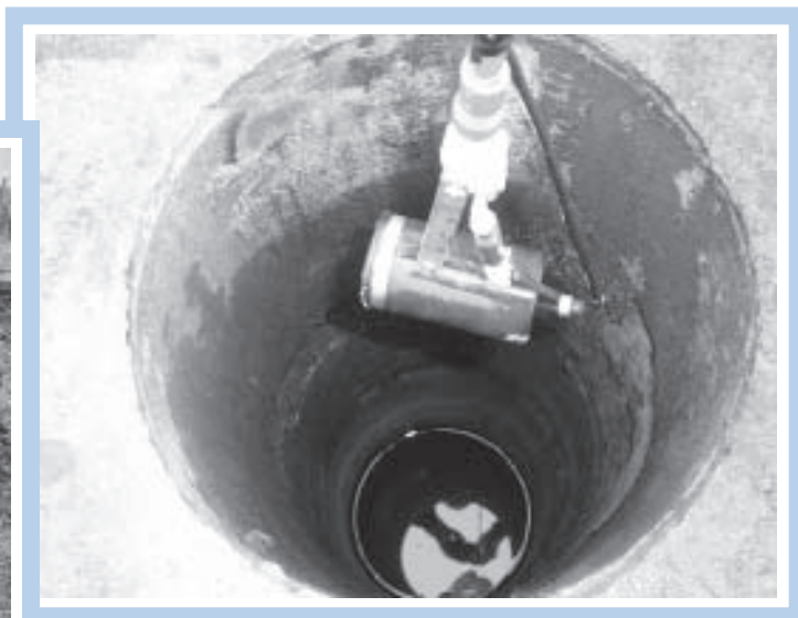
Figure 4. Underwater camera about to be lowered into a well to look for problems in the casing and screen.
