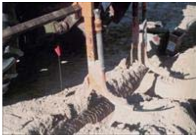
View of a drain plow used to install subsurface drip irrigation tubing.
