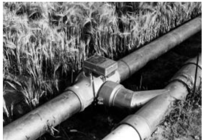
Surge flow system. The surge controller is shown.
