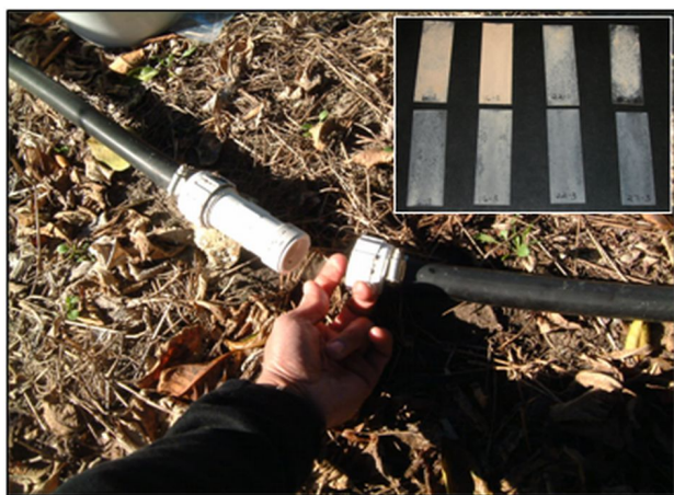
Figure 5. A 3/4-inch PVC coupling found in plumbing-supply stores serves well as in-line glass slide holder. Observing the amount, type, and rate of scale deposition occurring on a clean side (inset) can help determine the scaling potential of the irrigation water and the effect of injected scale-inhibiting chemicals.
