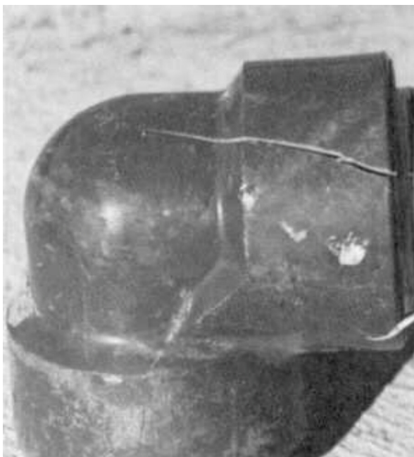
Figure 4. Example of threaded PVC fitting failure due to ever-tightening (reprinted with permission from Bliesner, 1987).
