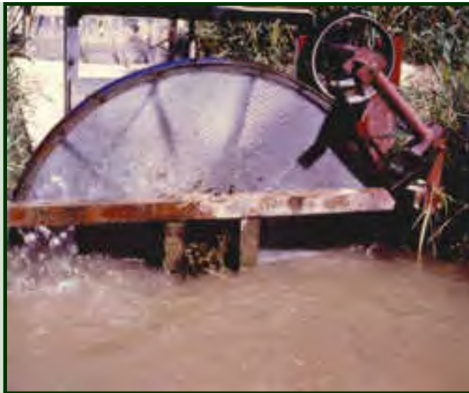
An electric-powered wheel screen at a canal entrance. Click on image to enlarge.
