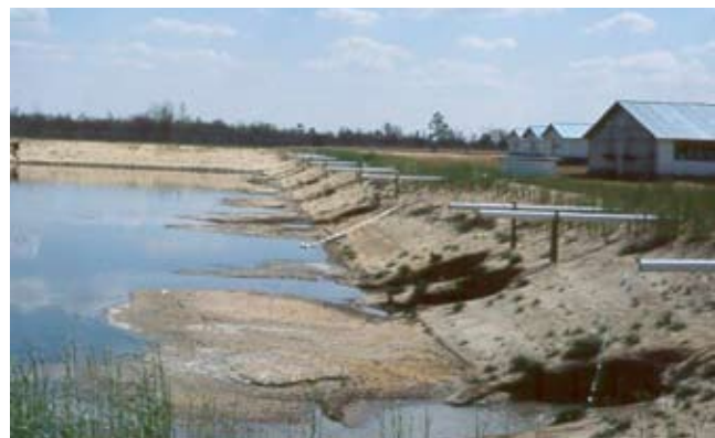
Figure 10D–21 Old agricultural waste storage pond constructed before modern standards were placed in effect
