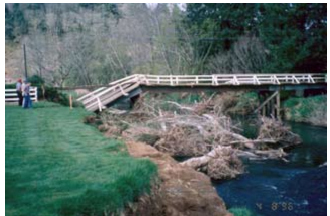
Figure TS14Q-2 Flood-damaged bridge in EWP program (Photo courtesy of Ben Doerge)
