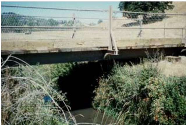
Figure TS14Q-1 Farm bridge with steel I-beam structural members and timber strip footing (Photo courtesy of Ben Doerge)
