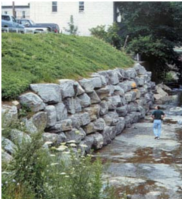
Figure TS14D-15 Reinforced soil slope with rock face (Photograph courtesy of Frank Cousin, NRCS MI)
