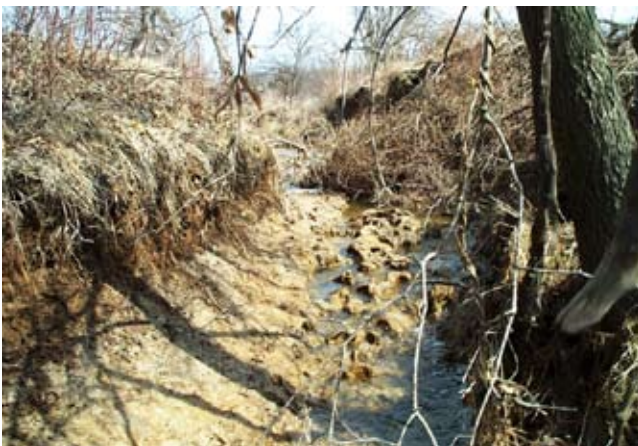
Figure 2-11 Systemwide downcutting induced by channelization project downstream. Additional landowners must become involved to address the root cause of channel incision to stabilize the entire degrading reach. This is an example of a threshold or flow-driven stream. (Hurricane Creek, Jefferson County, IL)
